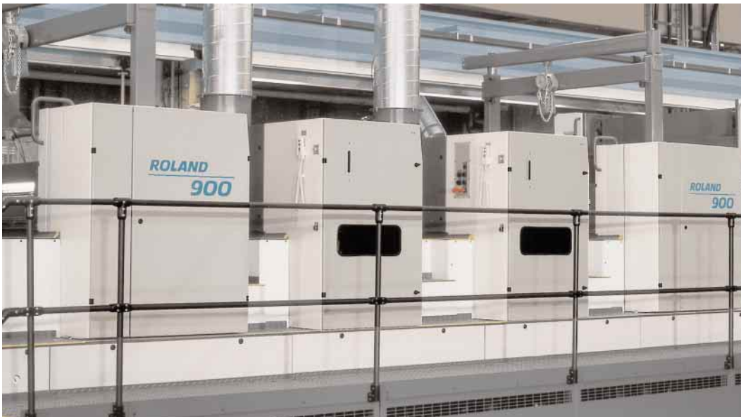
The double coating module with its dryer systems is centrally controlled from the central control console.
